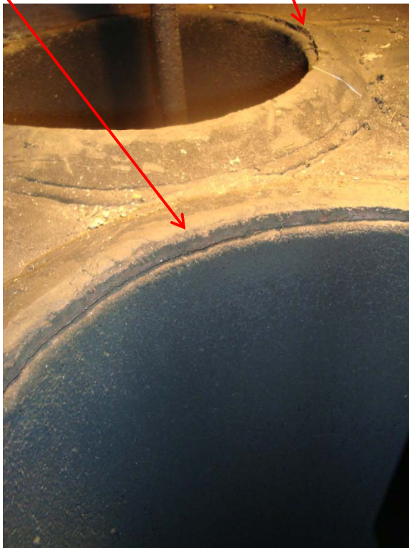
Deformed and cracked collector pipes
